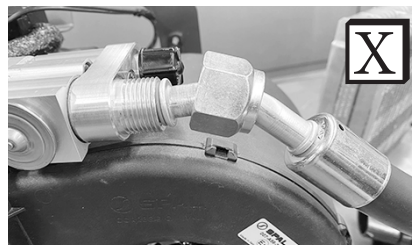
Improperly Seated O-ring Land
